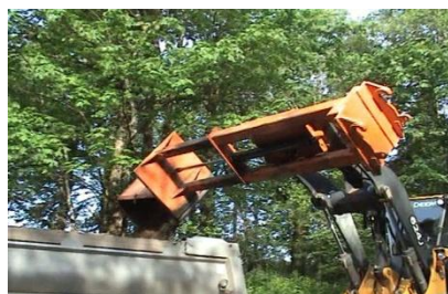
After dumping the debris, you can return to the ditch and repeat the process.
